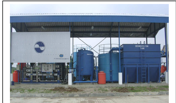
Water Recycle Plant PT. Chemco Harapan Nusantara - Karawang
