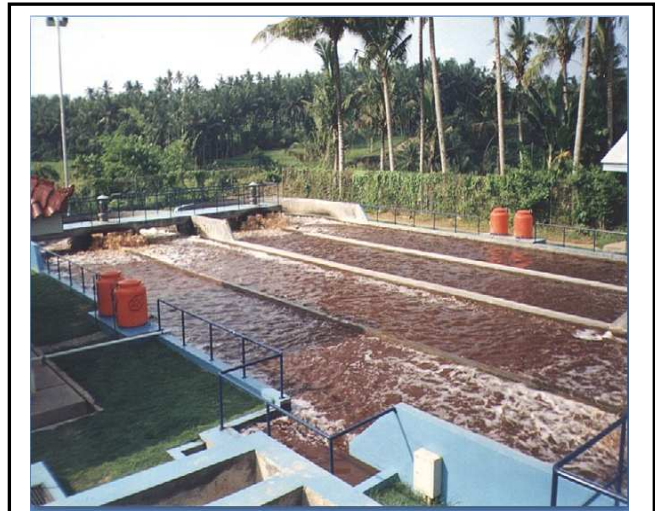
Waste Water Treatment Plant PT. SINAR SOSRO – BALI
