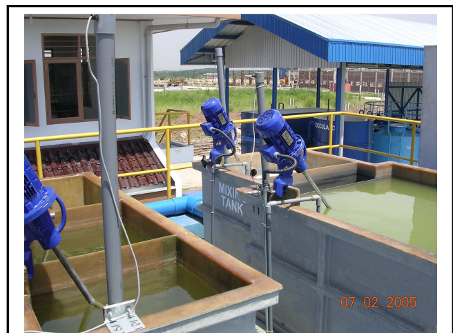
MIXING TANK PT. CHEMCO HARAPAN NUSANTARA
