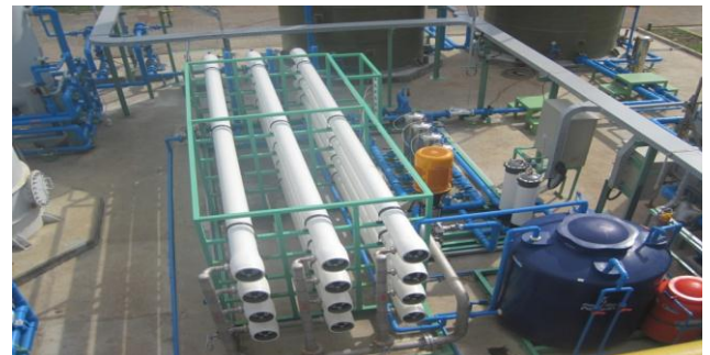
PT ASAHIMAS CHEMICALS (ASC) - CILEGON Year of construction :2011 Capacity : 56 m 3 /hour
